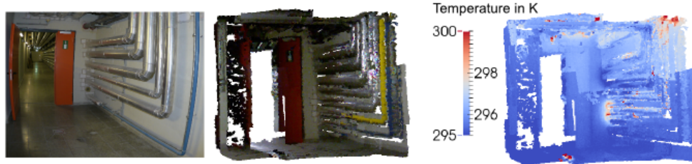
Figure 12. Second 3D-representation of a utility corridor 2. Left: Picture of the place. Middle: Visual-3D representation. Right: Thermal-3D representation.
