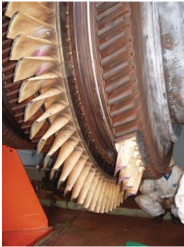
Fig. 1. A gas turbine system for electrical power production, under maintenance.
